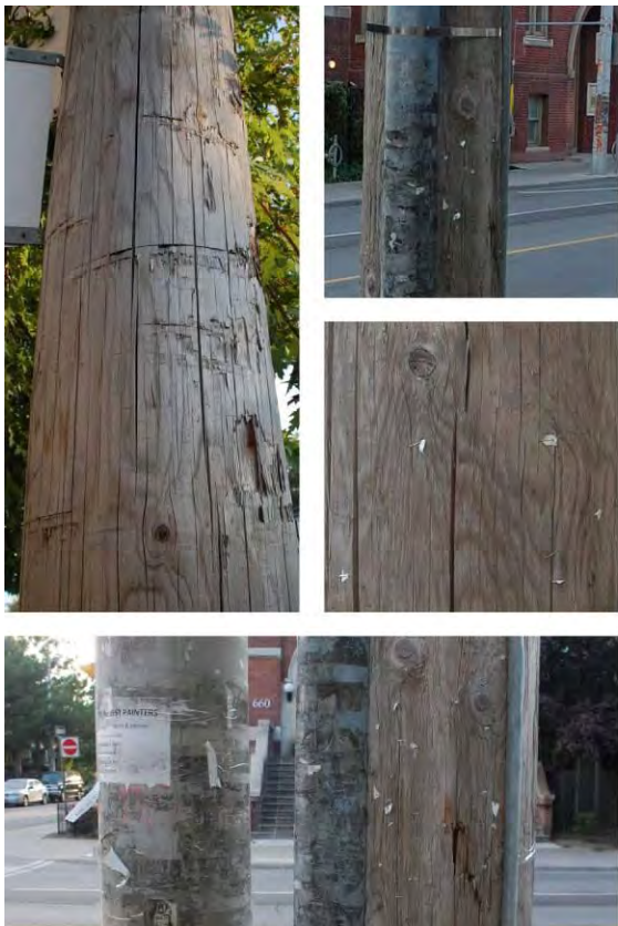
Lightly stapled & taped wood poles
