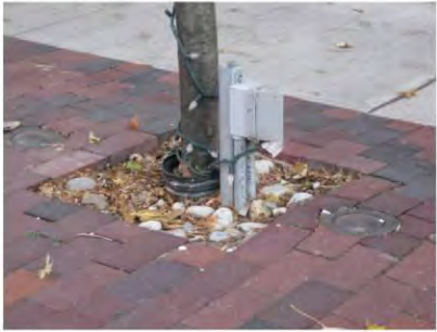
● Seasonal Lighting Power (Distillery District) 15A, 120V receptacles to power light strings
