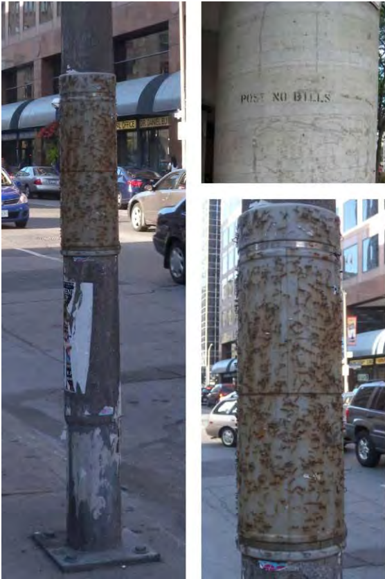
Pole-mounted devices – Church Street
