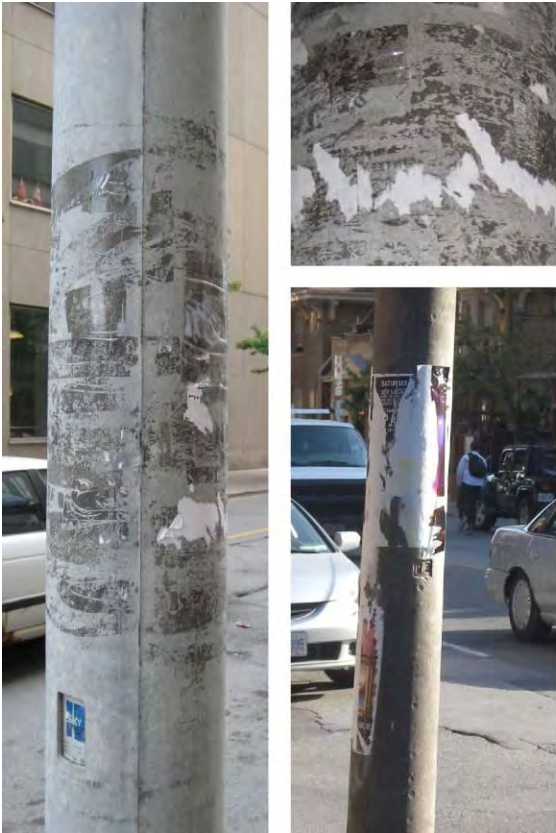
Adhesive residue on concrete poles
