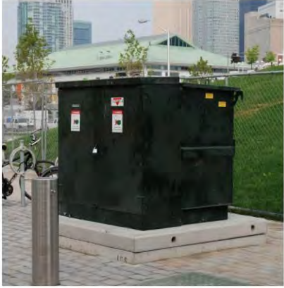
SG Pad-mounted Switchgear (Sugar Beach) 1.4m x 1.4m exterior dimension 5.4m x 3.4m clear required
