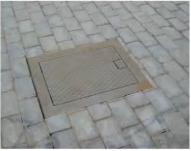
■ In-ground Electrical Receptacle / Event Power (WEP) 0.8m x .06m surface dimension
