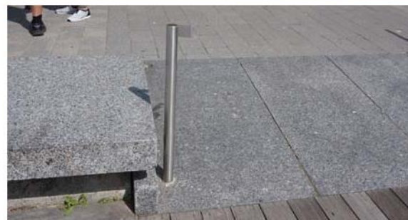
Reference: broken handrail at York Quay
