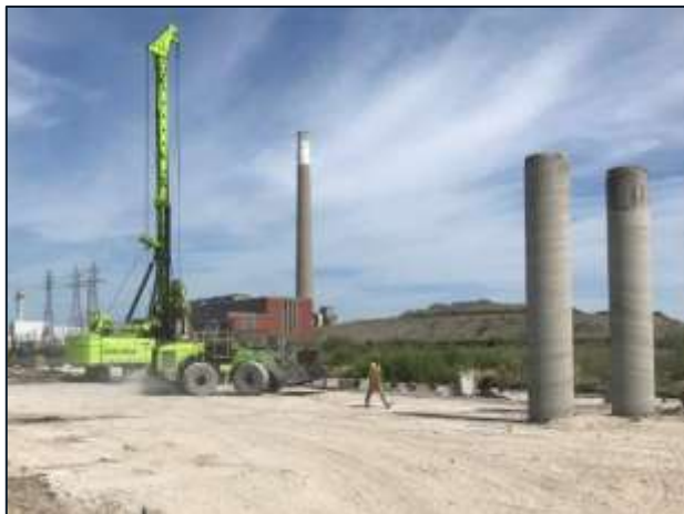
New River Valley – Secant wall construction ongoing at north and south end of the river valley.
