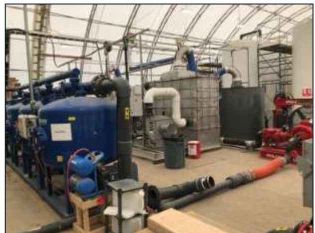
Water Treatment Plant – Treatment operations ongoing.
