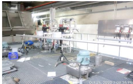
Inside at the Flocculation Tanks
