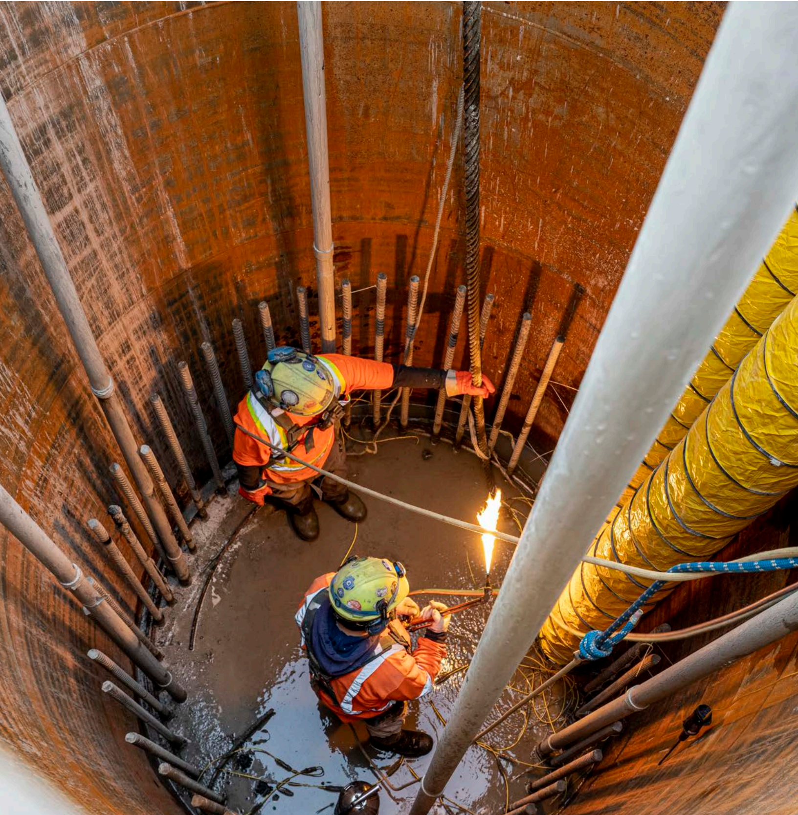
A crew completes work on part of the Cherry Street South Bridge foundation. See page 60 for more on the family of four bridges that will connect Villiers Island to the mainland. Image by Vid Ingelevics and Ryan Walker.
