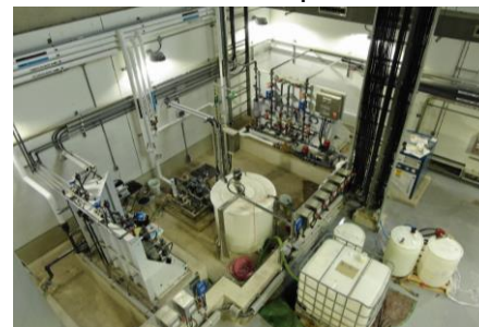
Inside at the Chemical Tanks
