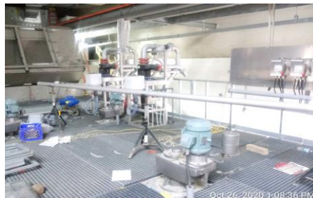
Inside at the Flocculation Tanks
