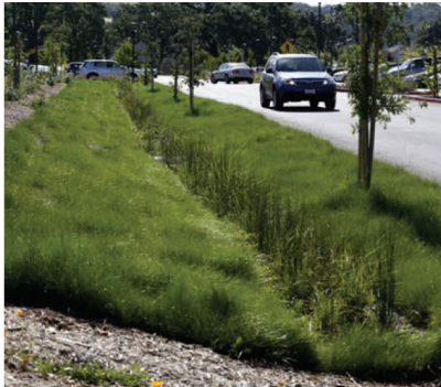
1A Enhanced grass swale
