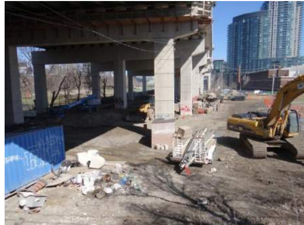
Plate 2: The study area under the Gardiner Expressway showing construction activities, facing east
