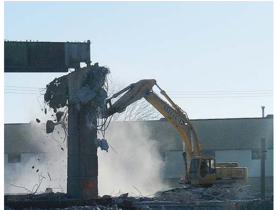
Demolition of the Gardiner structure to the east of the Don River. 1999. (source: City of Toronto)
