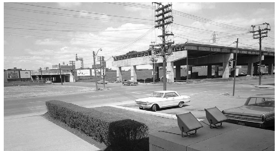
Jarvis Street, east side, looking northeast from Lake Shore Boulevard East, showing Gardiner Expressway under construction. 1963. (source: City of Toronto Archives)
