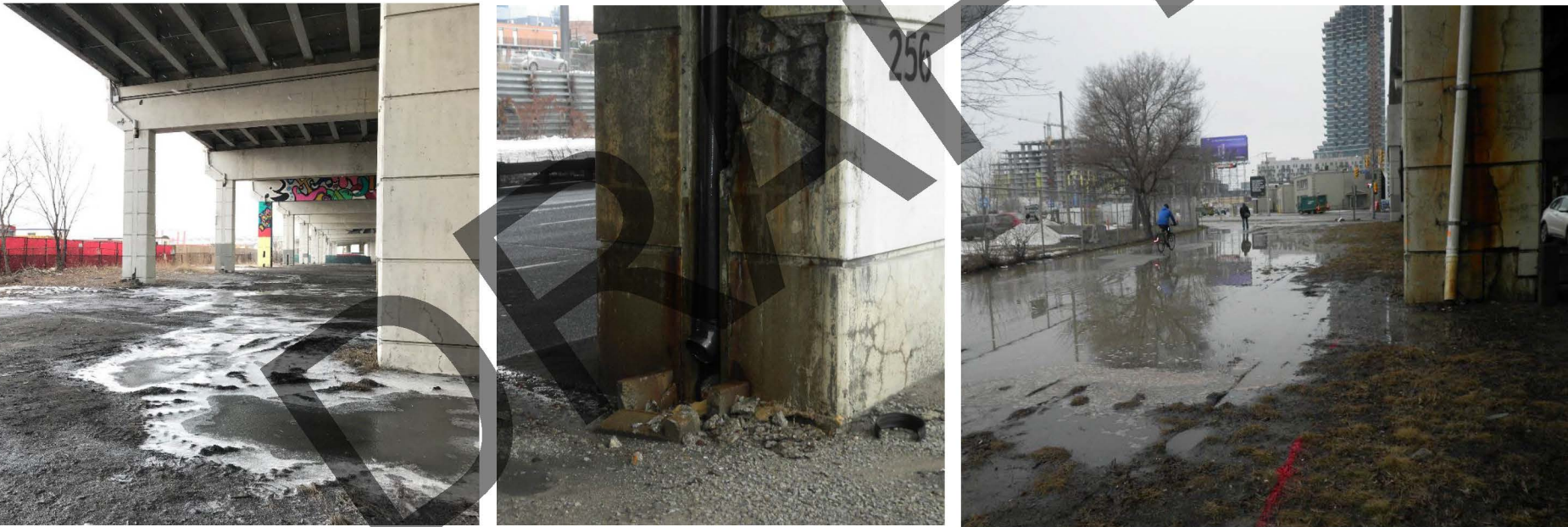
EXISTING CONDITIONS: SURFACE PONDING IN CONFLICT WITH PEDESTRIANS
