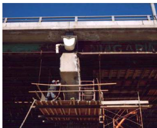
Bent repairs required.
