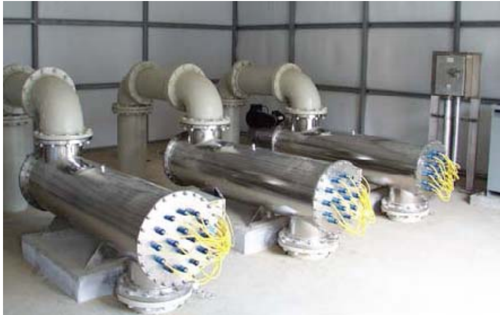
Figure 5-12: Ultraviolet Disinfection System
