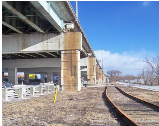
Railway Spur line runs beside Lake Shore Boulevard east bound lane from Cherry Street to Parliament Street (looking east, just east of Parliament) – since decommissioned
