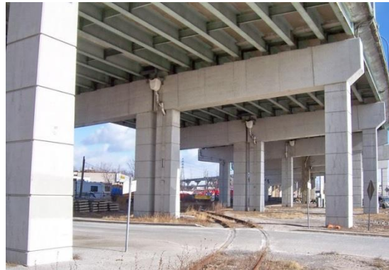
Abandoned railway spur line under the Gardiner Expressway and crossing LSB to the Metrolinx Don Yard (looking east).
