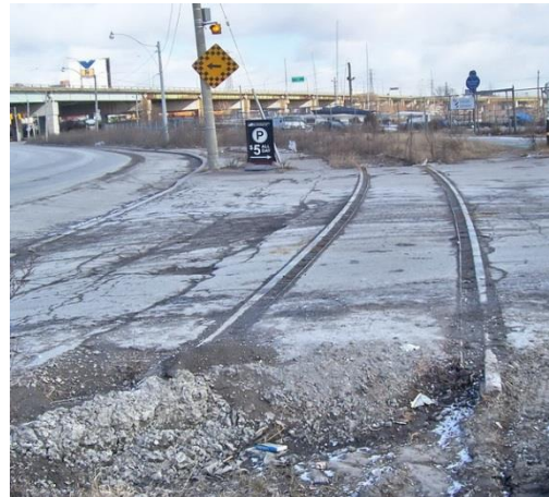
The Spur Line dead ends approximately 250m south of Lake Shore Boulevard at Parliament Street. There are isolated areas that have abandoned tracks in place, Redpath Sugar, LCBO warehouse
