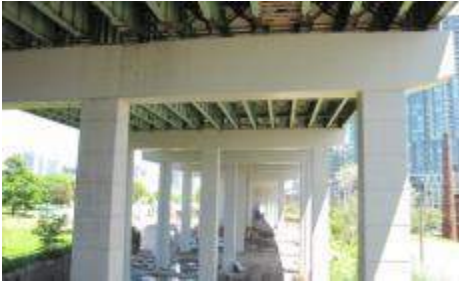
KEY IDEA – Rehabilitated Infrastructure: Rehabilitating the existing columns and girders of the Gardiner East. (Gardiner Expressway at Fort York).
