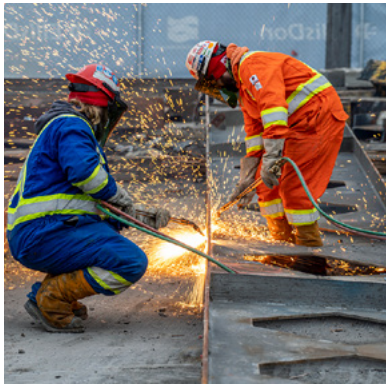
Construction at the Port Lands: Welders working on the reclaimed metal girders from Marine Terminal 35. The girders will be used as guard rails on the new bicycle bridges in the parks.
