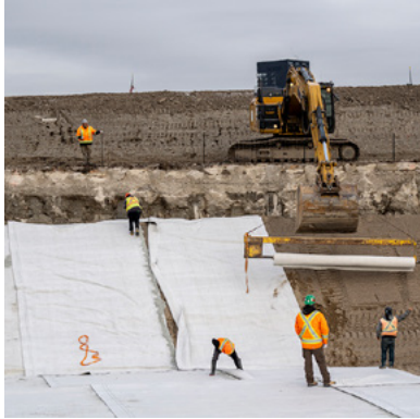
Construction at the Port Lands: Crews installing geosynthetic clay line. Along with geomembrane and protective sand, the liner provides a barrier between the soil below the river and the river bottom finishes.
