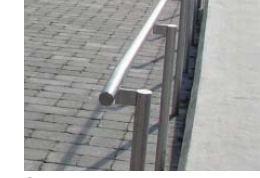
Stainless steel handrail
