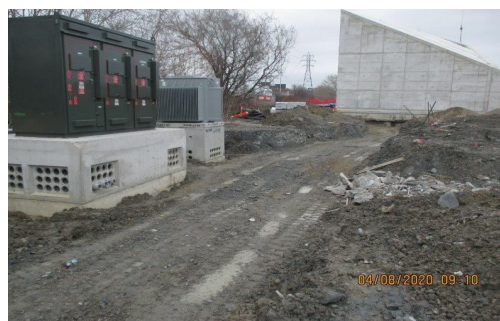
SWF Electrical equipment
