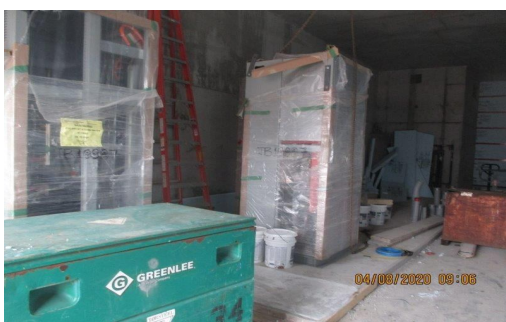
SWF Electrical room
