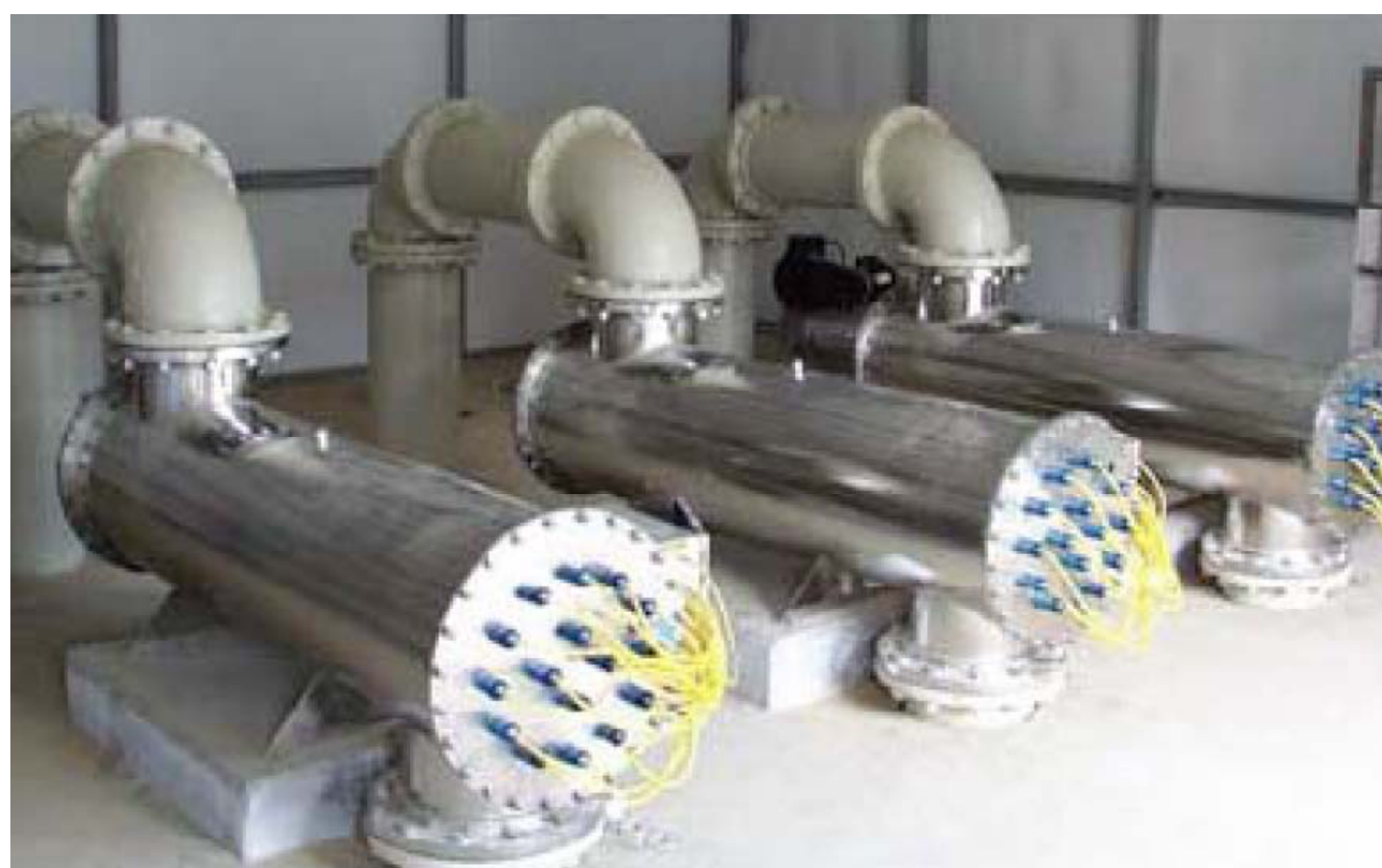
Ultraviolet disinfection system
