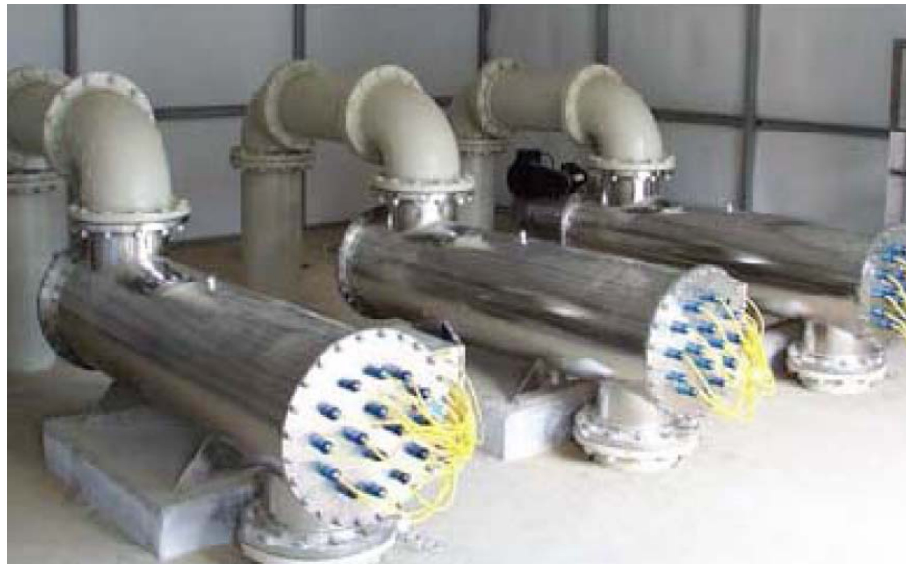
Ultraviolet disinfection system
