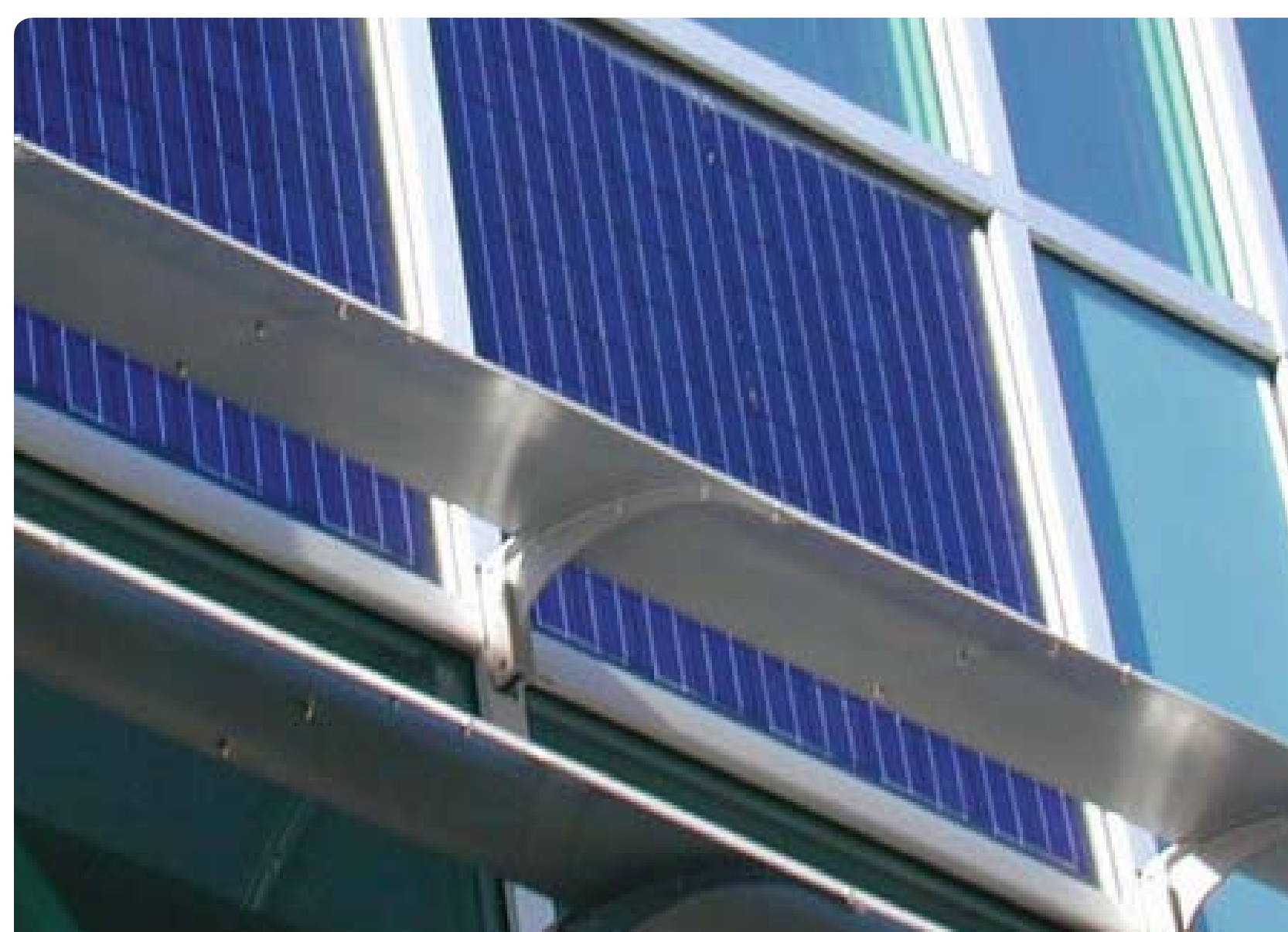
Solar paneled facades and sun shades on south building faces
