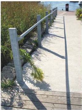
GALVANISED METAL RAILING ALONG BOARDWALK EDGE.
