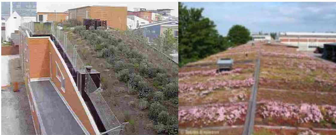
Figure 3:8 Stormwater Flows can be considerably decreased by a Series of Control Measures, here exemplified by Green Roofs, Ponds and Wetlands.
