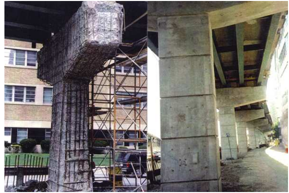
The Poor Condition of the Existing Gardiner Must Be Addressed.
