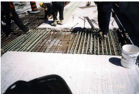
Deck Replacement Will Be Necessary to Prolong the Life of the Existing Structure.
