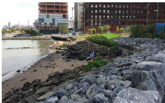
FIGURE 3-3: Example of exposed armouring
