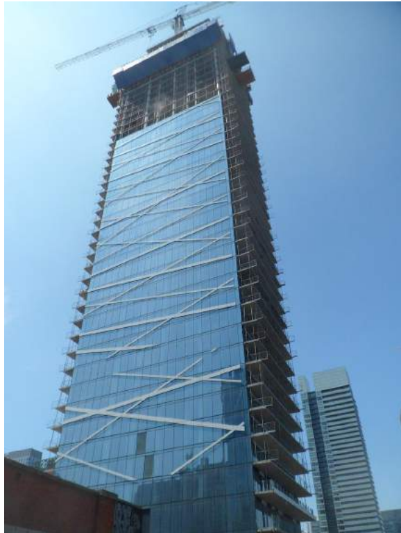
Figure 7.6 High window-to-wall ratio and curtain wall system, Theatre Park Condos, Toronto (Image Credit: Urban Toronto)
