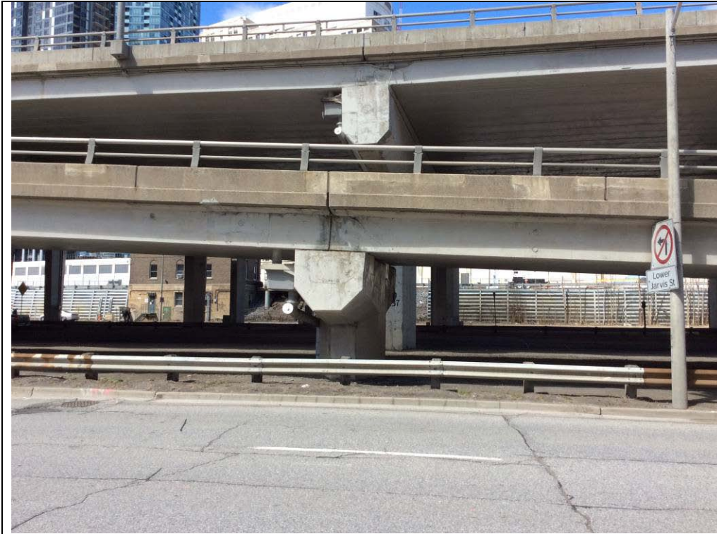
Plate 11: Detail of the concrete pier supporting the superstructure of the Gardiner Expressway off-ramp.
