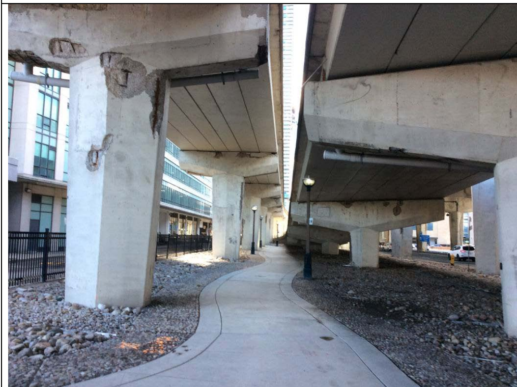
Plate 12: View of the pathway beneath the Gardiner Expressway off-ramp, looking west from Yonge Street.
