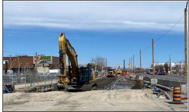
Figure 6 Lakeshore Blvd (North Side) - Booth to Carlaw - Installation of Dewatering System Completed
