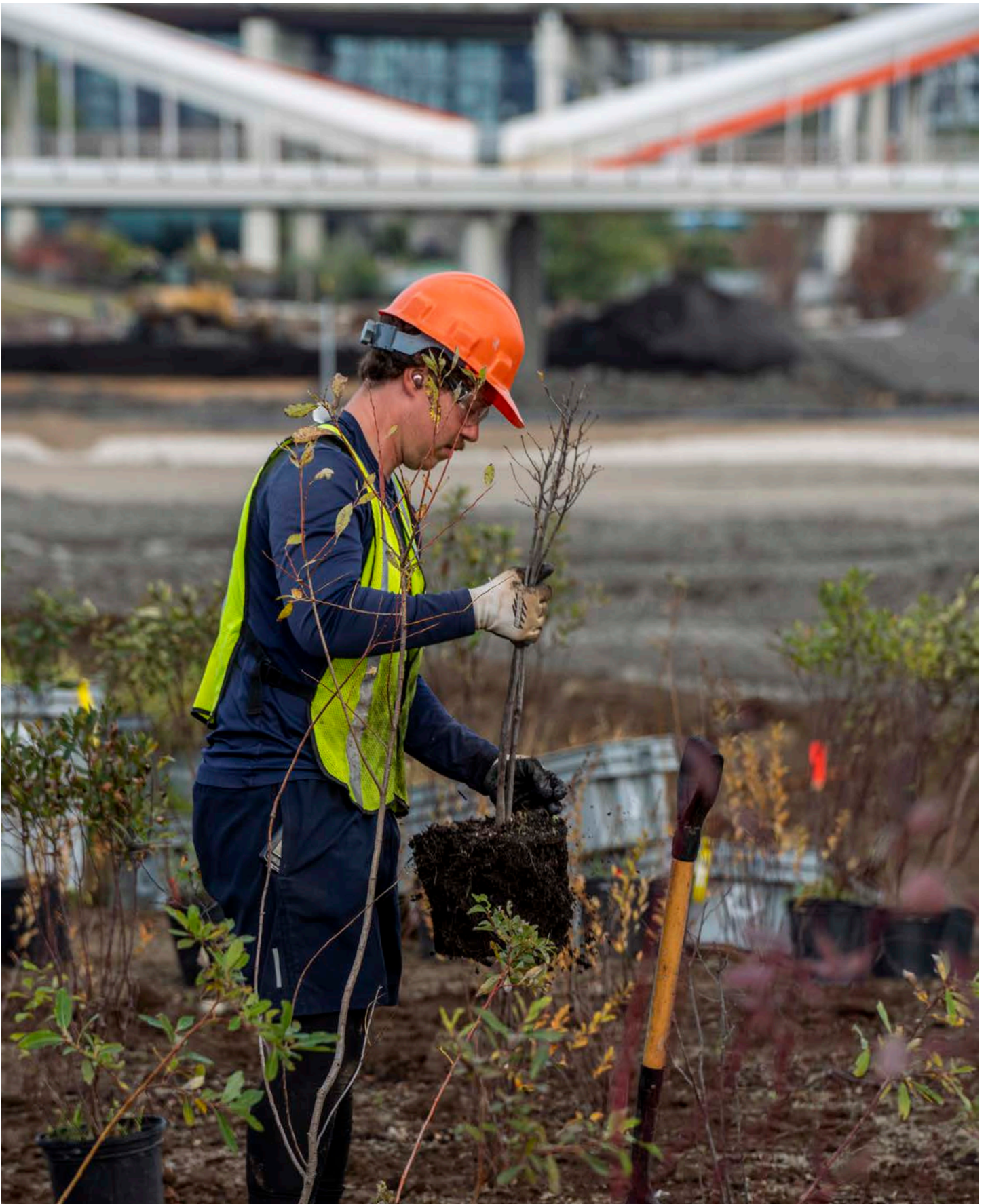
Most of the millions of plants being established in the marshlands in the new Don River Valley must be planted by hand. Image by Vid Ingelevics and Ryan Walker.
