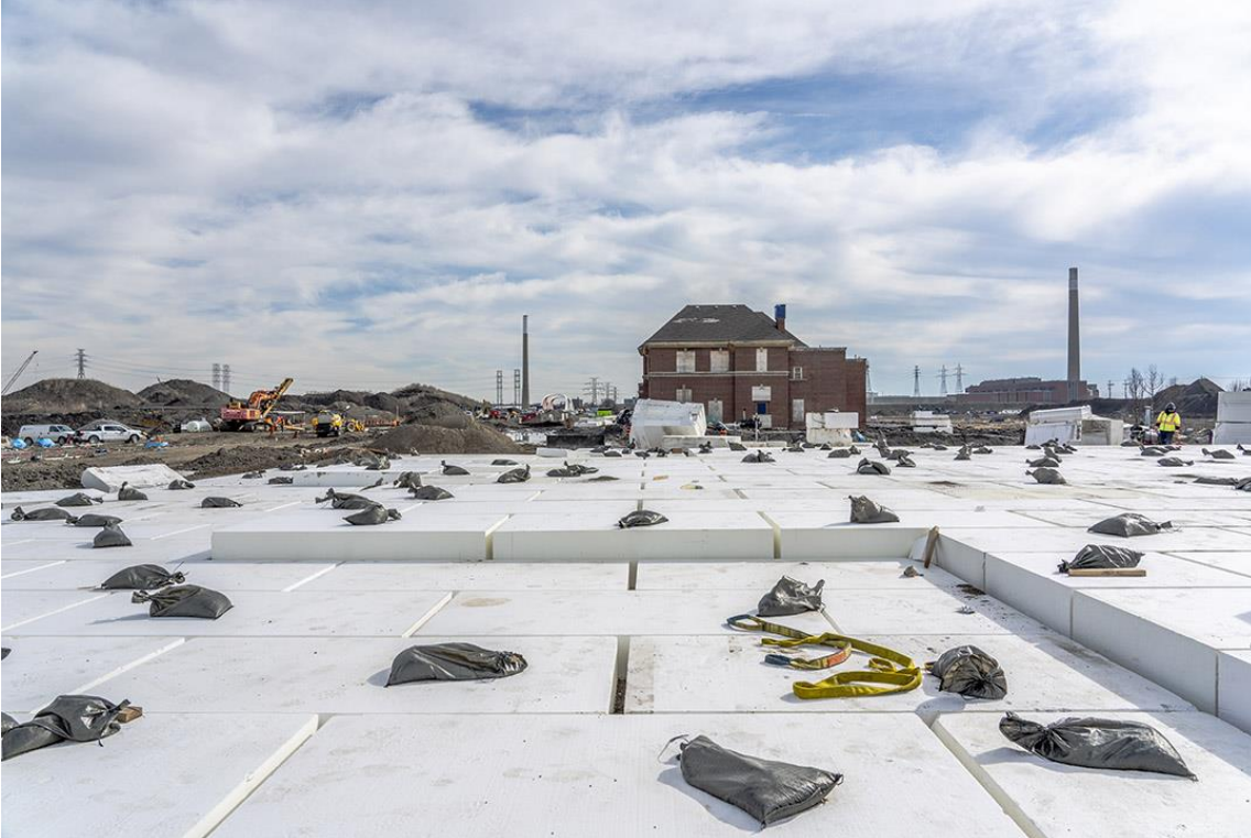
Above: These large white blocks are geof foam in future River Park North. This lightweight material is placed in the ground above infrastructure like pipes to avoid putting too much weight on them. Then the geof foam is covered with soil.
