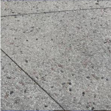
Exposed Aggregate Concrete with granite aggregate and special saw cuts Intersection corners
